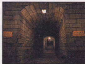
The sewers aren't big enough to get lost in, but watch out for the street access sign.
